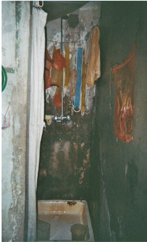
Figure (8) the poor condition of the cell walls and moistness on the sides of the wall is most clear.
